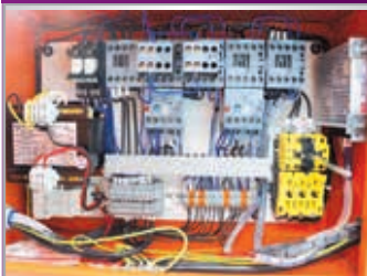
DC control cabinet
